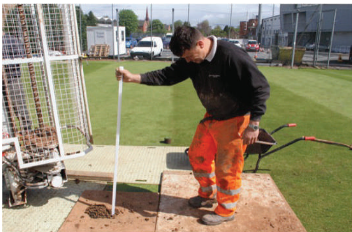
The EGRP ® system installation is a low impact design versus the traditional excavation methods that tear up land. The system is installed by our professional Certified Parjana ® Installers. Most installations take less than one week to complete depending on site conditions and solution requirements.
